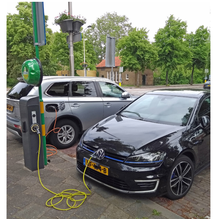
Figure A2.8b: Electric vehicle charging station (Francis Flinch - Own work, CC BY-SA 4.0, https://commons.wikimedia.org/w/index.php?curid=79231008 )
