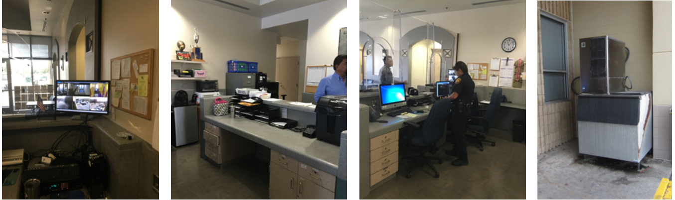
Service Agent Area @ Central, Ice Machine example (required at exterior at Park Police facilities)
